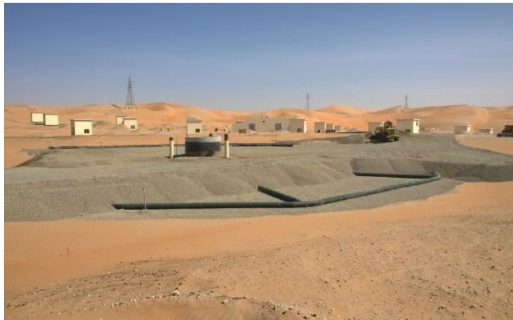
FIGURE 1: REALISATION OF A SUBSURFACE INFILTRATION BASIN WITH 105 ASR WELLS IN THE LIWA DESERT.
