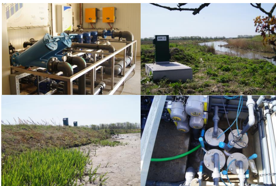
FIGURE 2: IMPRESSION OF THE ASR WELL FIELD IN AN ECOLOGICAL CORRIDOR IN THE GREENHOUSE AREA
